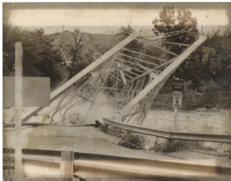
Destruction of the 1878 Pratt Truss Bridge by Hurricane Agnes in 1972.
